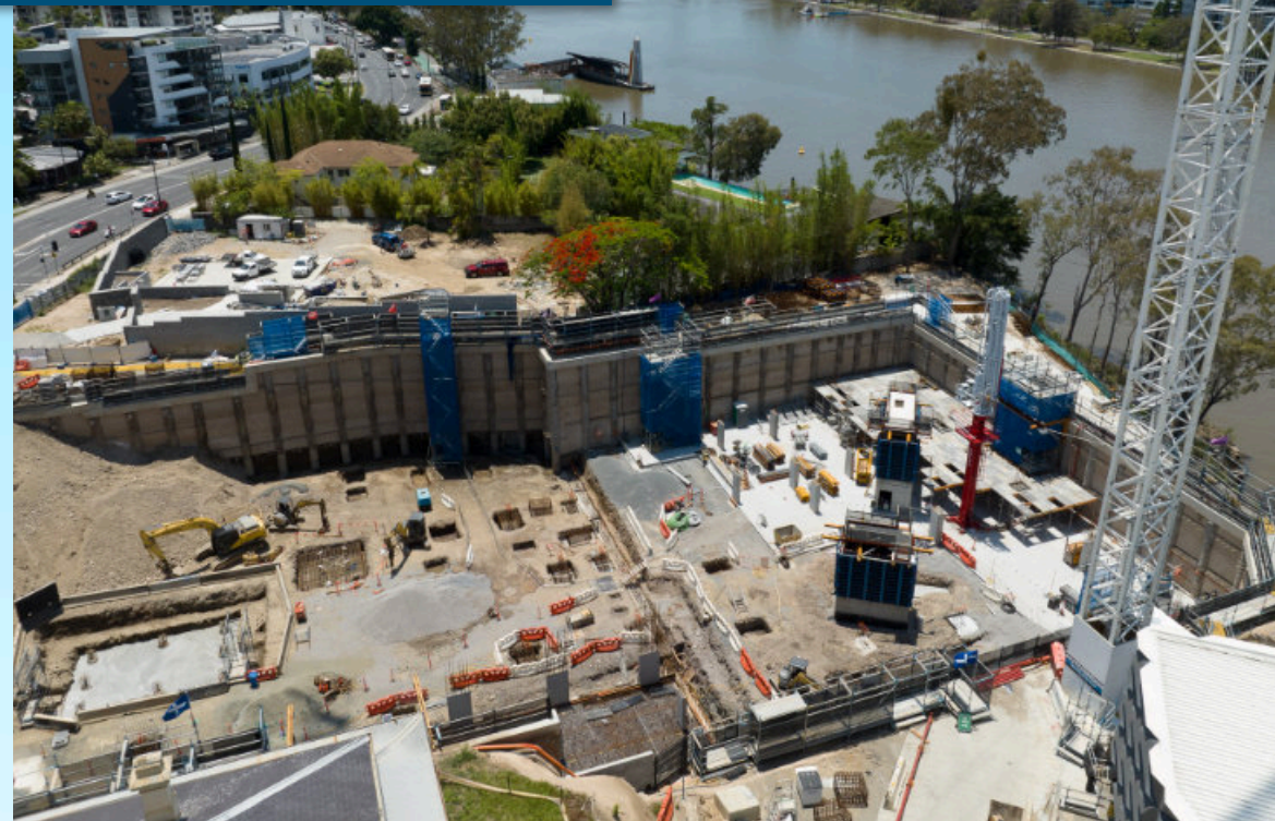
Stunning city and river views appear as Monarch's twin towers emerge simultaneously from the prime riverside site at Toowong.
